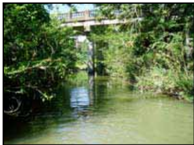
Dry Comal Creek, urban stream located in the city of New Braunfels
